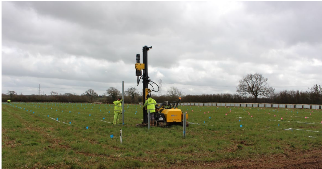
Plate 11a: Marking out location of the infrastructure and installation of Mounting Structures (1 of 4)
