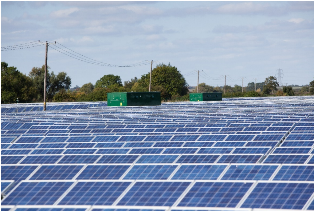
Plate 3: Example of Solar Station located within a PV Array
